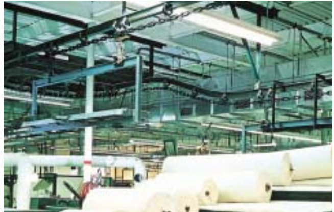
Trolley conveyor system
