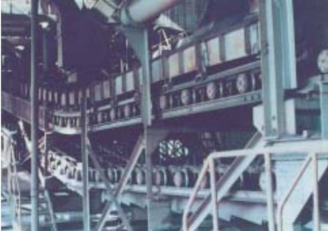
Long pan conveyor
